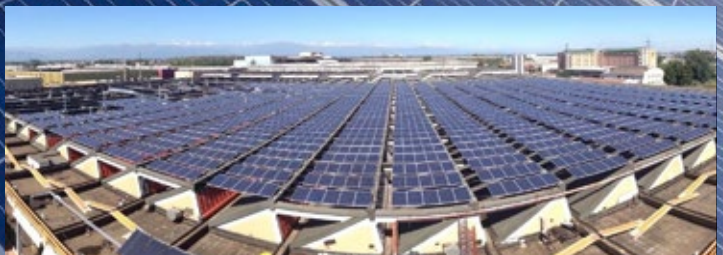
Commercial rooftop solar power plant
